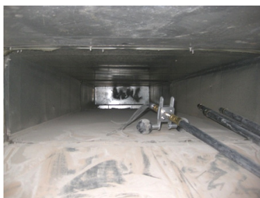
Filthy Ductwork before being cleaned. Caked with dirt.
